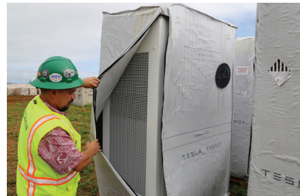
Image Credit: Katie Fehrenbacher for Fortune TESLA'S SOLAR BATTERY FARM FORTUNE: https://goo.gl/uiTZV9 PBN: https://goo.gl/OfV3cu SOLARCITY: https://goo.gl/AbC3KH
